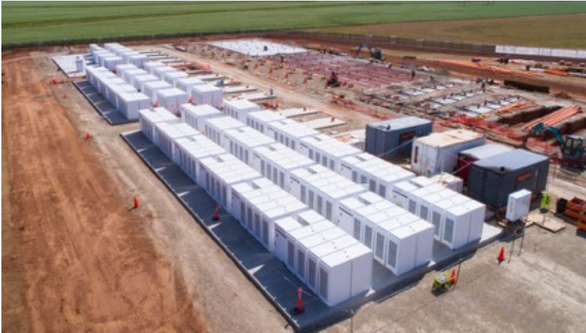
Figure 7: The Hornsdale Power Reserve (South Australia) in the process of expansion from 100 MW/129 MWh to 150 MW/193.5 MWh, as of November 2017.
