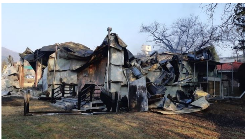
Figure 2: Remains of a Korean BESS destroyed by a “battery fire”. An energy storage system was destroyed at the Asia Cement plant in Jecheon, North Chungcheong Province, on Dec. 17. Courtesy of North Chungcheong Province Fire Service Headquarters (Korea Times 2 May 2019)
