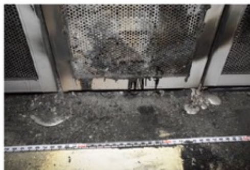
Figure A.1: Photograph taken during decommissioning of the ESS shows a pool of solidified aluminum on the floor in front of Rack 15 [1].
